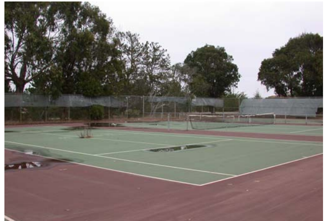
Existing tennis courts should be refurbished
