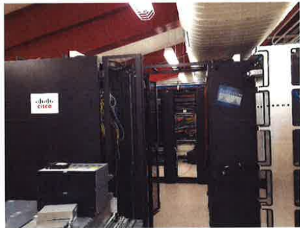
Figure 63: Server room equipment and ventilation duct
