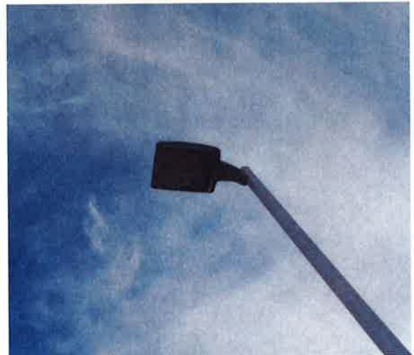
Figure 34: External HID lights at Seaside Public Safety
