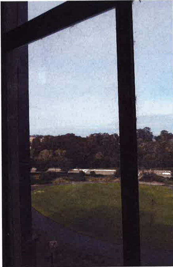
Figure 23: Dirty exterior pane of windows in Library
