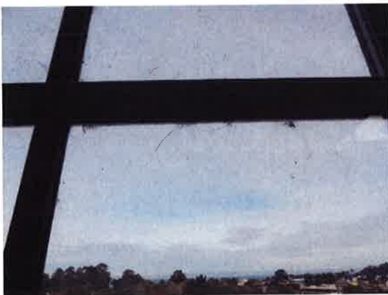
Figure 25: Dirty exterior pane of windows in Library
