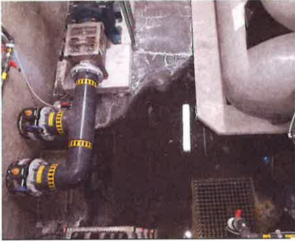
Figure 46: Faulty sump pump in pool pump house.
