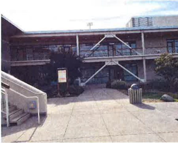
Figure 49: North elevation view of Student Services Building with awnings and exterior lighting constantly on.
