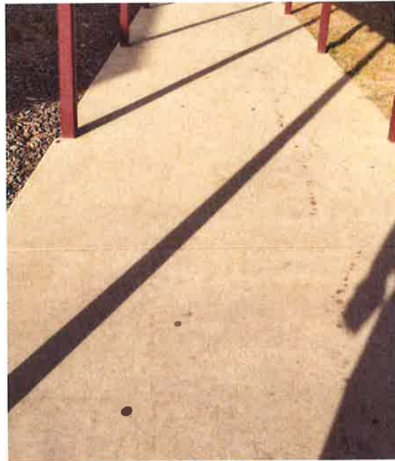
Figure 73: Stained pavement under covered walkway at entrance to Marina Center
