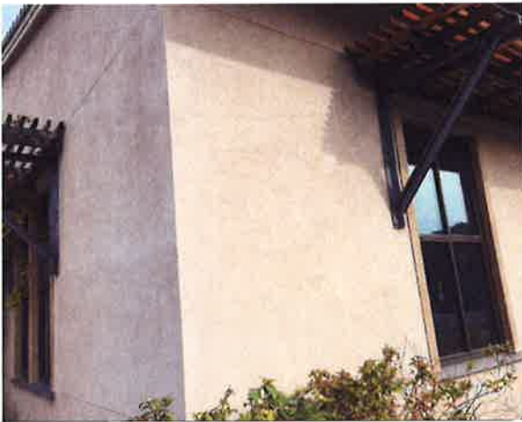
Figure 45: Stucco cracked and repaired at entrance to Library
