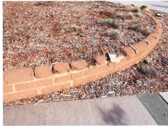
Figure 53: Damaged raised flower bed wall at General Classroom Building
