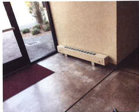
Figure 30: Water hammer was noted in radiant heater on 1st floor in Gym
