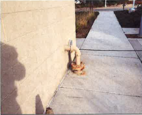
Figure 43: Corrosion starting to show on exterior of steel water pipes at Seaside Public Safety
