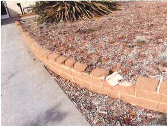
Figure 52: Damaged raised flower bed wall at General Classroom Building
