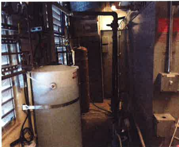
Figure 48: Clean & tidy Physical Science Building boiler house
