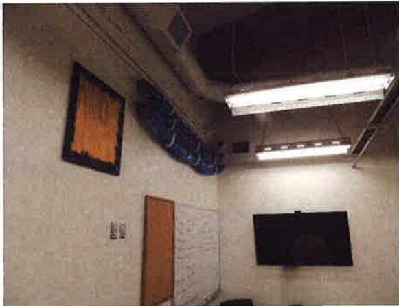
Figure 62: Fireproofing of server room cables
