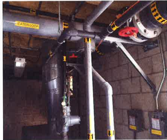
Figure 47: Labelled valves and pipework in pool pump house.
