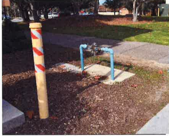
Figure 44: Leaking backflow valve assembly outside Art Gallery
