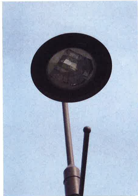
Figure 32: Exterior "Spanish Lamps" with HID lighting scheduled for replacement with LED heads.
