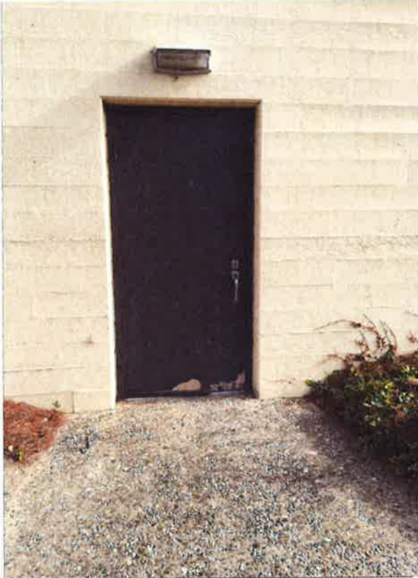
Figure 4: Damaged door at Lecture Forum
