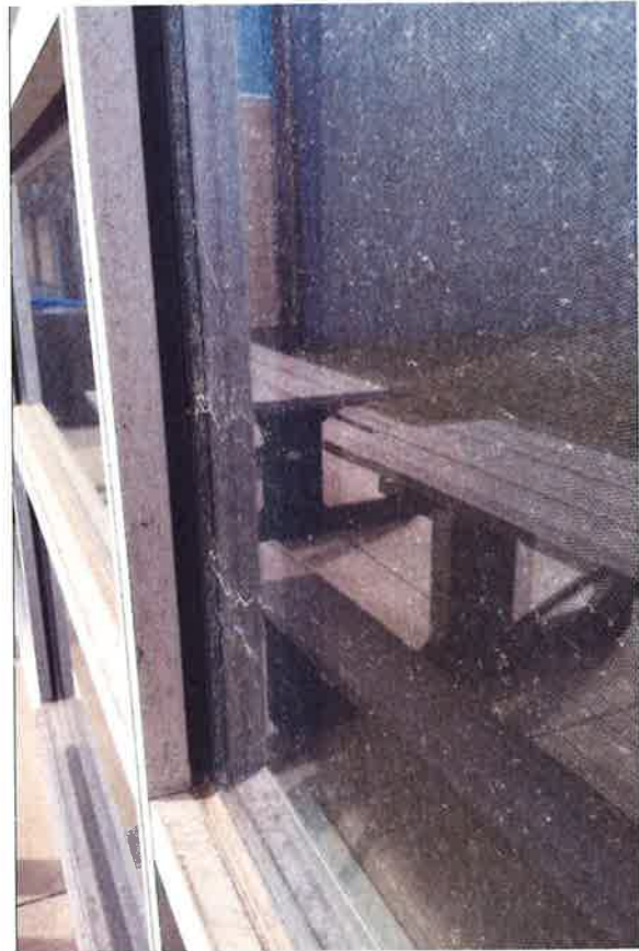
Figure 24: Dirty exterior pane of high-level windows in Marina Center
