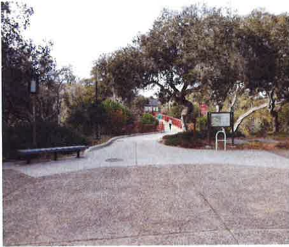
Figure 68: Bridge walkway and new pavement meeting cracked & uneven pavement outside Lecture Forum
