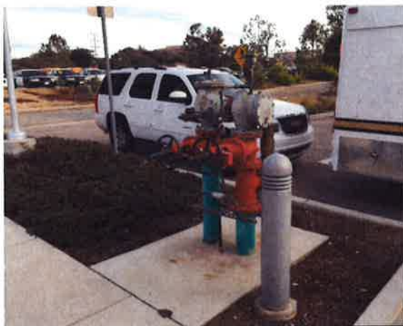
Figure 41: Primed and painted backflow and isolation valves and pipework at Seaside Public Safety Center
