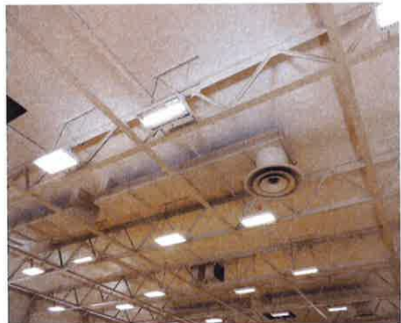
Figure 36: High-bay level fluorescent lighting in field house
