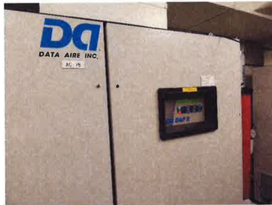
Figure 65: Computer Room Air Conditioning panel
