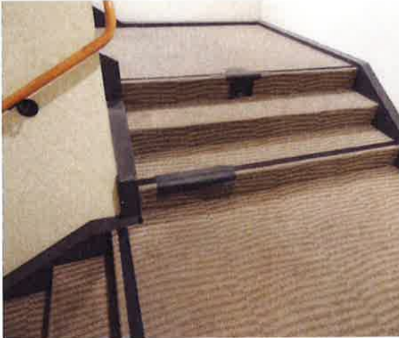
Figure 27: Stairwell carpet in Library needs attention
