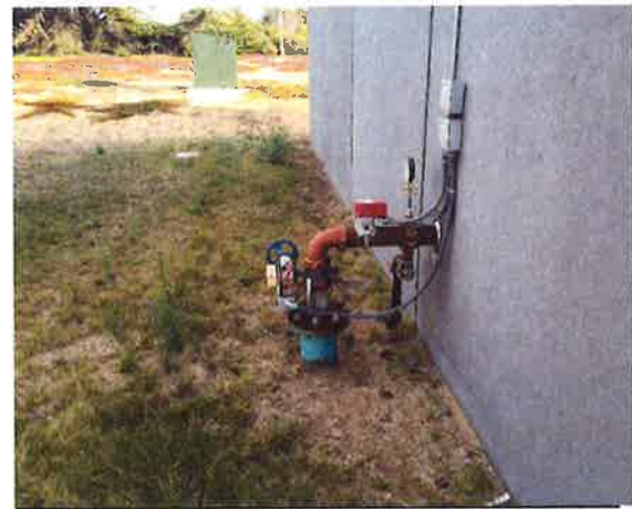
Figure 42: Steel water pipes corroding at Marina Center
