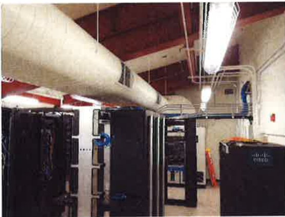
Figure 64: Server room equipment, ventilation ductwork and fluorescent lighting
