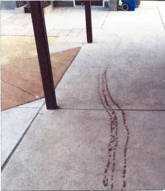
Figure 72: Stained pavement at Marina Center Courtyard
