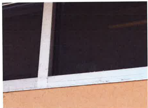
Figure 26: Dirty exterior pane of high-level windows in Marina Center
